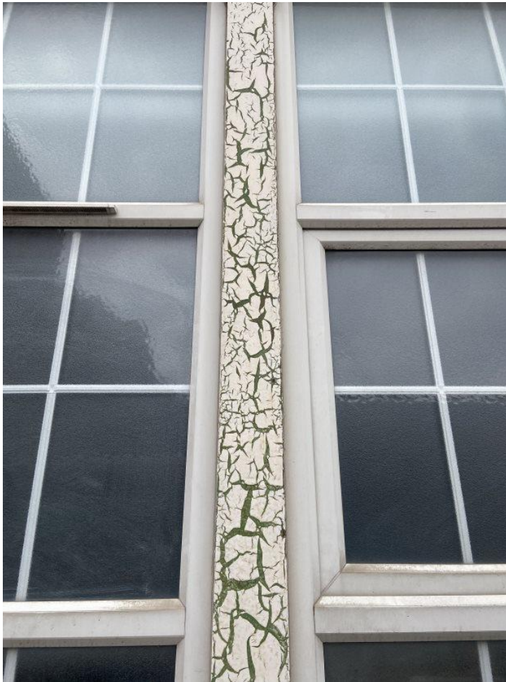
Figure 5.5 Low quality plastic glazing and poor decorative order have a detrimental significance on Berol House
