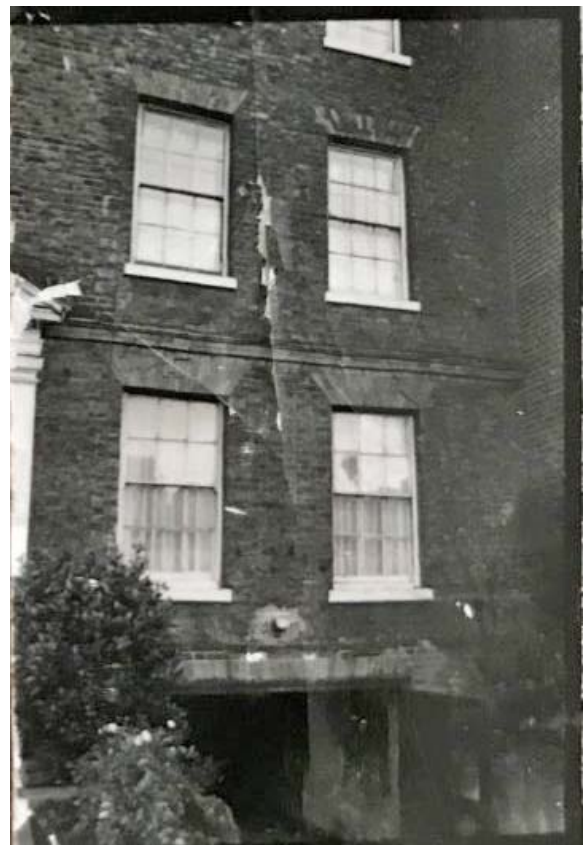
Figure 30 (Right) Number 794 in November 1977 showing the garage entrance in the front elevation. The extensive deflection and damage to first and second floor window arches indicates substantial movement occurred within this elevation.
