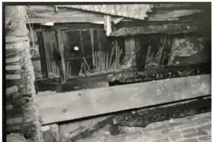
Figure 26 – The front rooms closest to Number 790 retained previous lathe and plaster but were extensively damaged.
