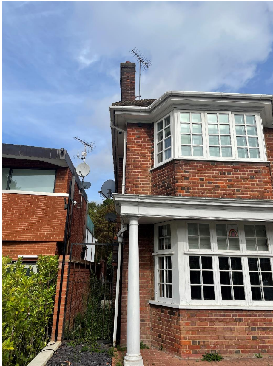
1.0 Leaning Chimney above Roof level
