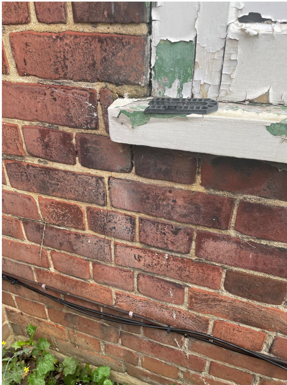
5.0 Cracking under ground floor window.
