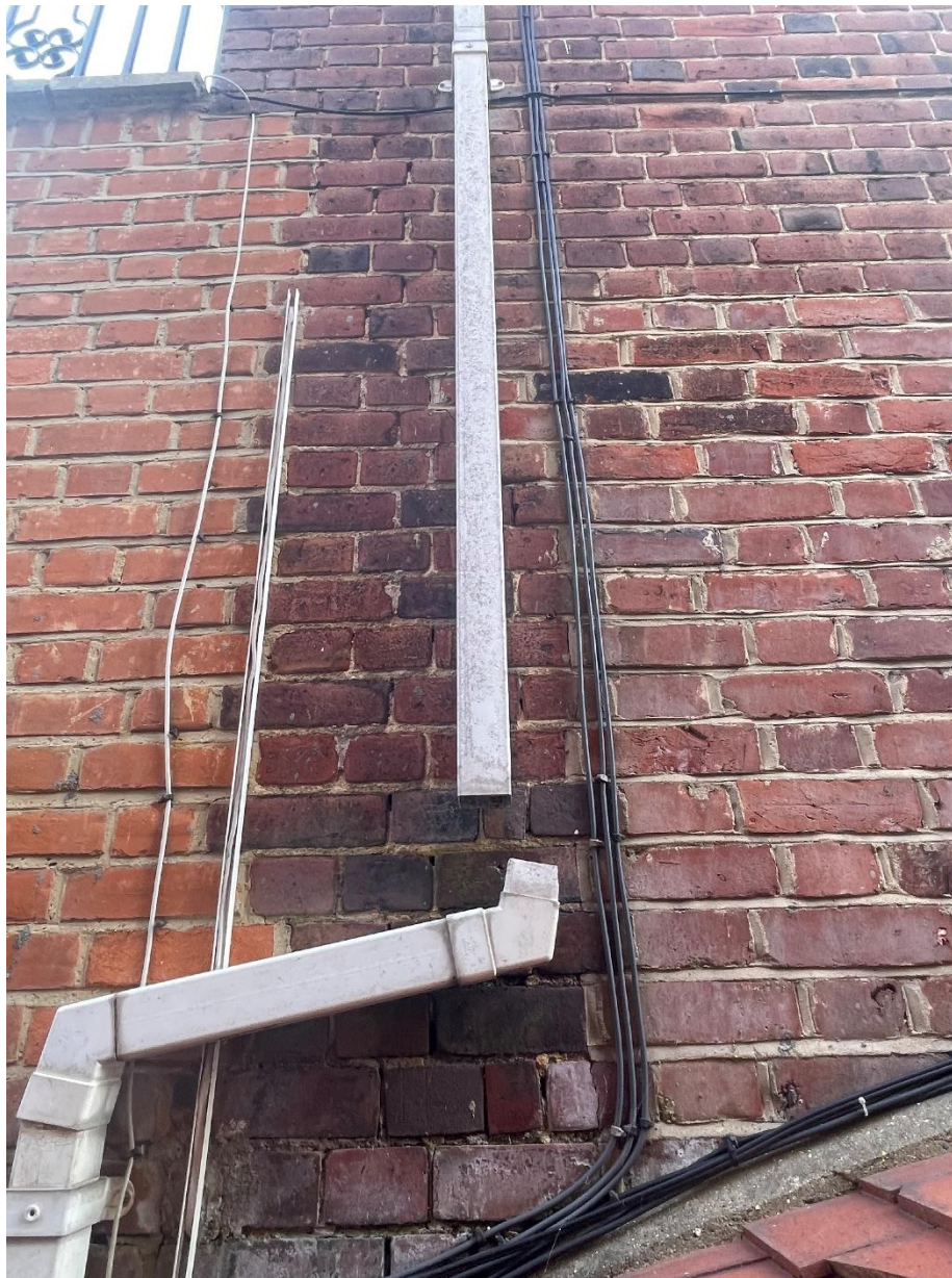
2.0 Cracking at toothed junction with newer extension. Questionable buttress.
