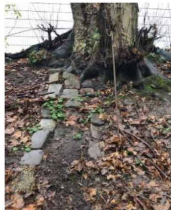
Fig. 14: One of the lateral pipe spillways into the ditch, blocked by tree roots
