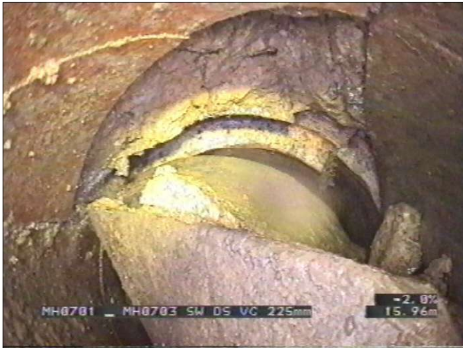
Photo: 8_29582a, Tape No.: 002, 23:59:42 15.96m, Hole in sewer from 09 to 03 o'clock Remark: obstruction broken pipe
