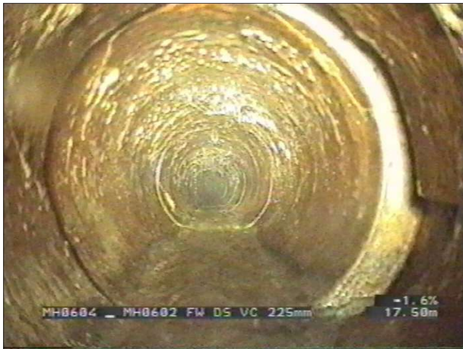
Photo: 5_5a, Tape No.: 002, 23:23:36 17.36m, Broken Pipe at joint from 04 to 06 o'clock
