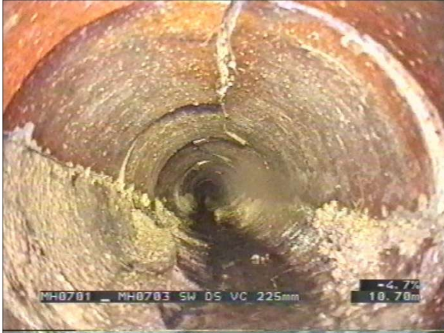
Photo: 8_29574a, Tape No.: 002, 23:58:57 10.76m, Broken pipe from 09 to 12 o'clock
