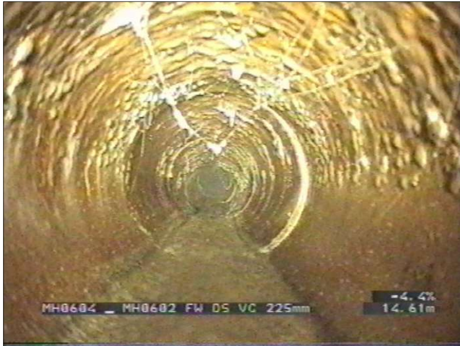
Photo: 3_3a, Tape No.: 002, 23:21:29 0m, Attached deposits, fouling from 09 to 03 o'clock 05 % cross-sectional area loss, Start
