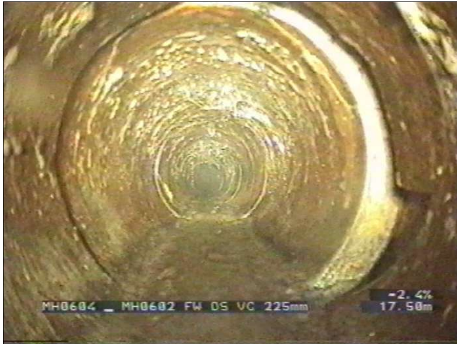
Photo: 5_5b, Tape No.: 002, 23:23:36 17.36m, Broken Pipe at joint from 04 to 06 o'clock
