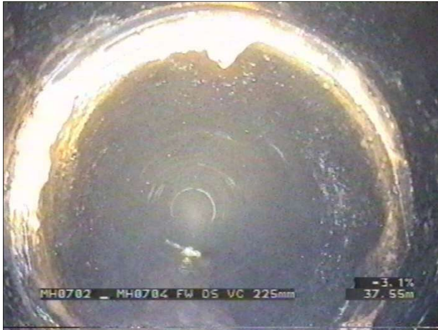
Photo: 58_3a, Tape No.: 002, 23:53:49 37.54m, Infiltration Dripping at 12 o'clock
