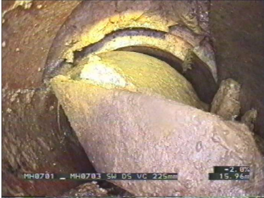
Photo: 8_29582b, Tape No.: 002, 23:59:42 15.96m, Hole in sewer from 09 to 03 o'clock Remark: obstruction broken pipe
