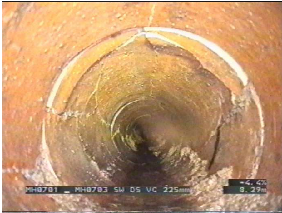
Photo: 8_29569b, Tape No.: 002, 23:58:36 8.42m, Broken Pipe at joint from 09 to 03 o'clock
