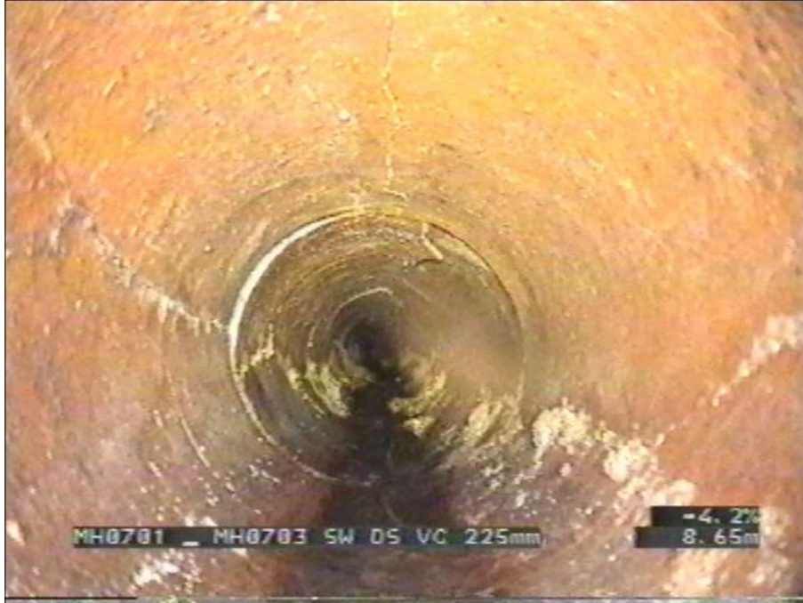
Photo: 8_29569a, Tape No.: 002, 23:58:36 8.42m, Broken Pipe at joint from 09 to 03 o'clock
