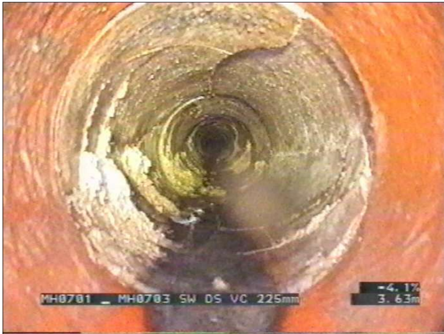
Photo: 8_29559a, Tape No.: 002, 23:57:43 3.76m, Fractures multiple from 10 to 06 o'clock
