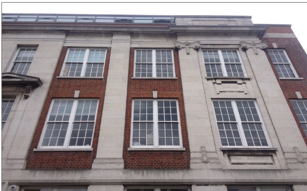
Existing stonework and brickwork requiring renovation
