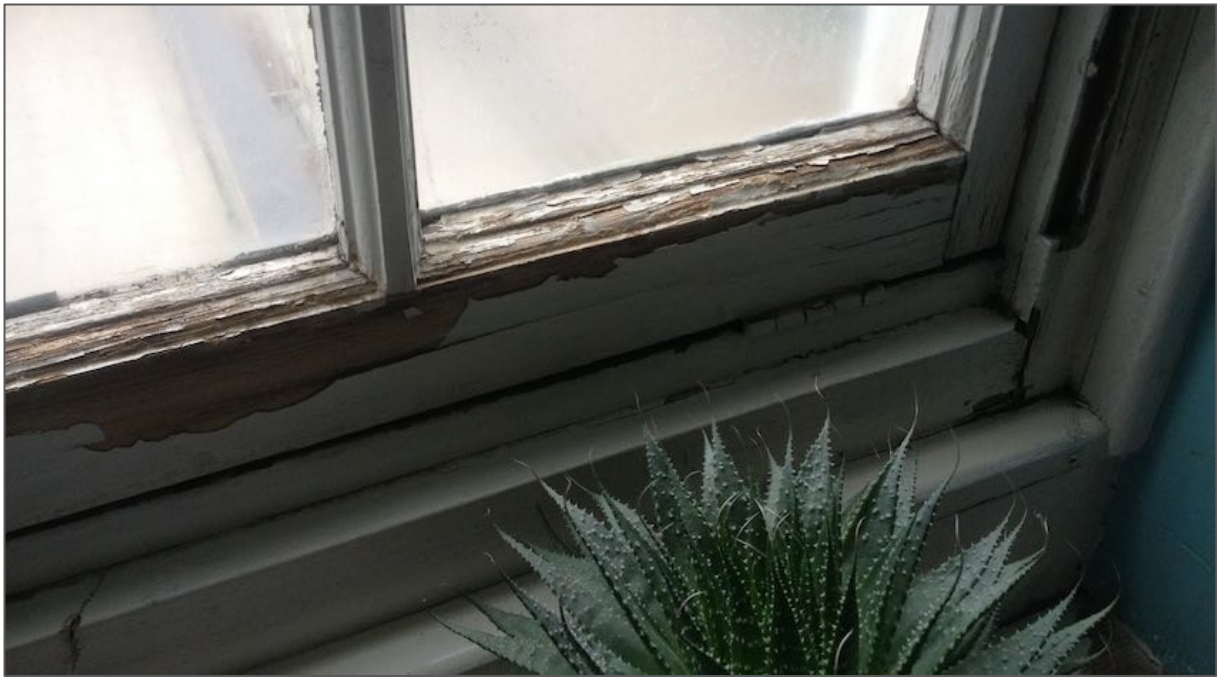
Existing damaged and poorly fitting windows to be replaced
