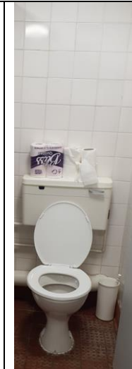
Image 14 Washroom Tiles and WC's
