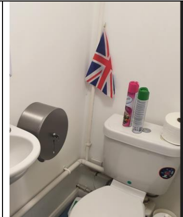
Image 18 Plasterboard Washroom Walls
