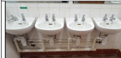
Image 15 Washroom Bathroom Basins
