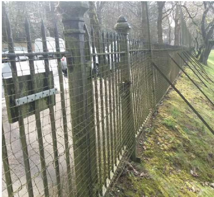
Fig. 6: Disused pedestrian access gate off Hampstead Lane
