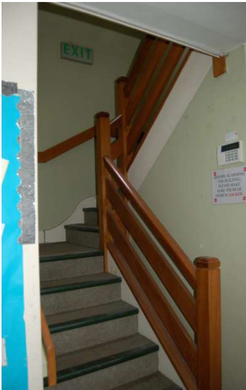
Restricted stair access
