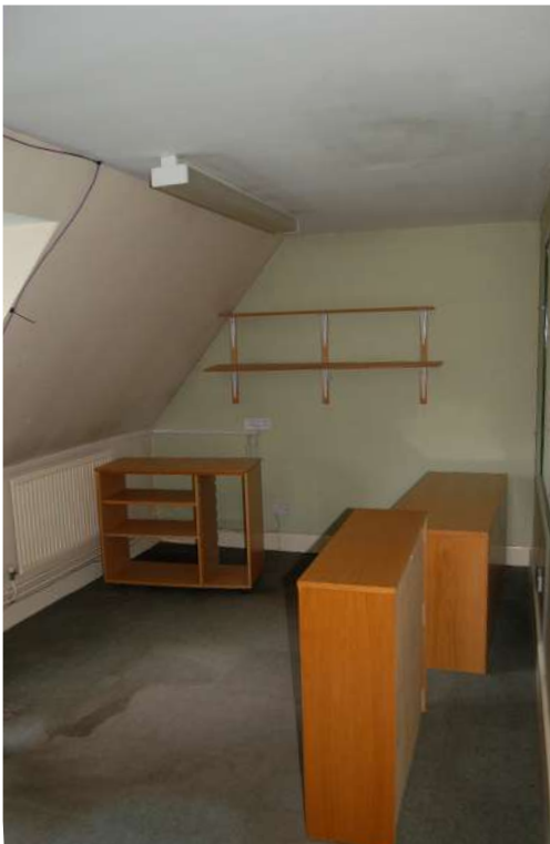
Extremely restricted headroom at first floor
