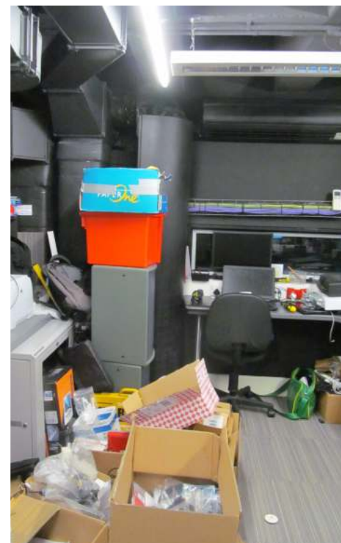
Inappropriate support facilities
