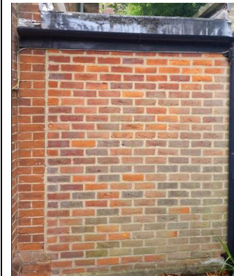
Image 3 External Brick Wall
