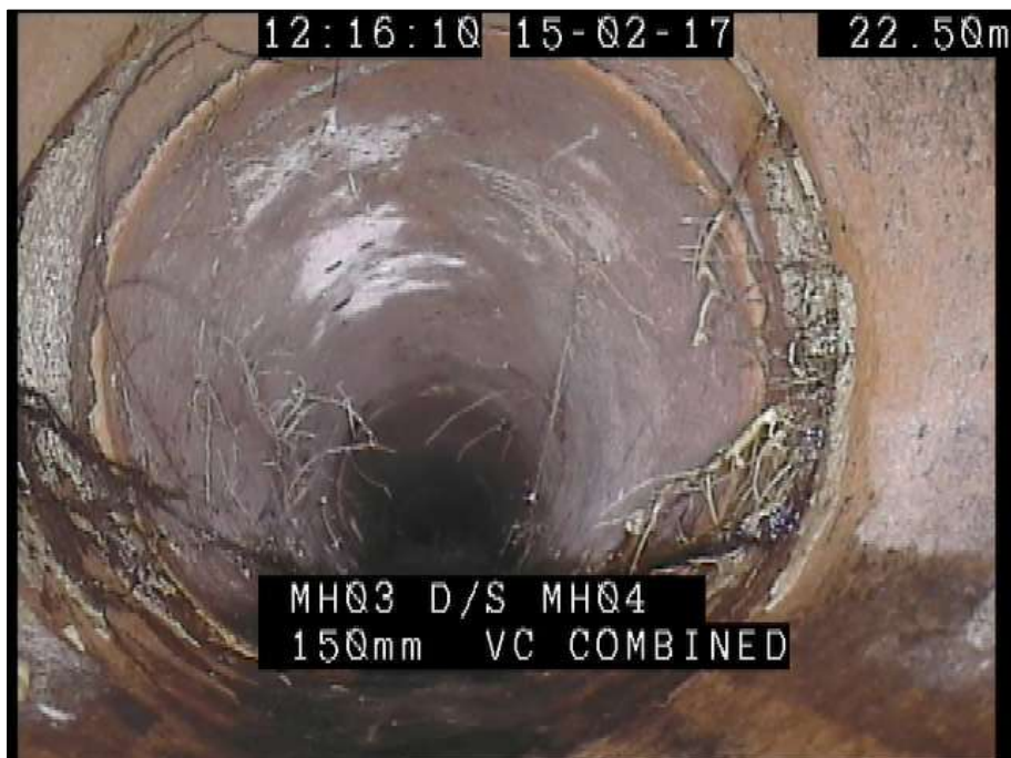
Photo: 4_11A 22.5m, Fracture, circumferential at joint, from 7 to 5 o'clock
