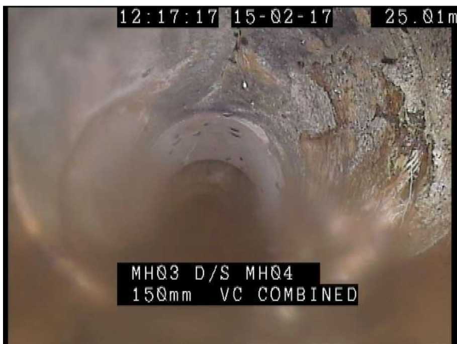
Photo: 4_14A 25m, Fracture, longitudinal, at 12 o'clock
