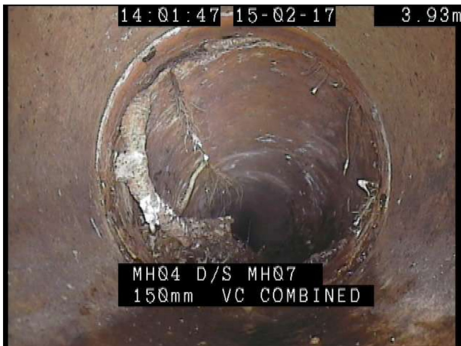
Photo: 8_7A 3.9m, Roots, tap Remarks: From break
