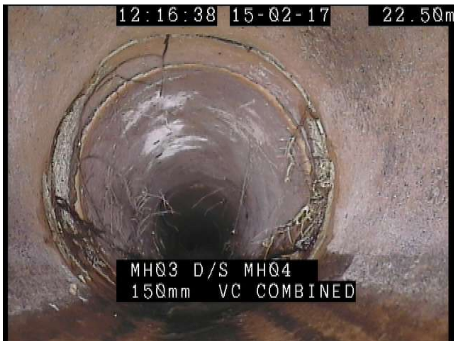
Photo: 4_12A 22.5m, Fracture, longitudinal at joint, at 12 o'clock
