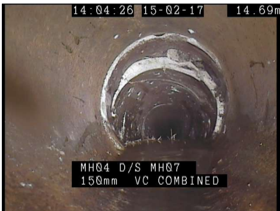
Photo: 8_12A 14.6m, Broken pipe, from 7 to 5 o'clock
