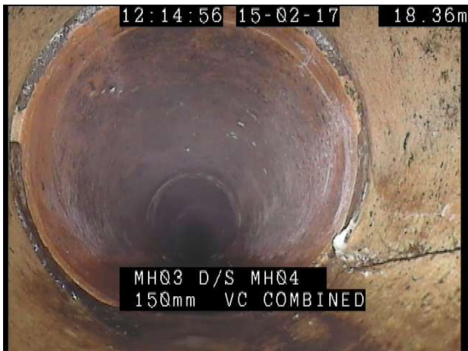
Photo: 4_8A 18.3m, Fracture, longitudinal, at 4 o'clock
