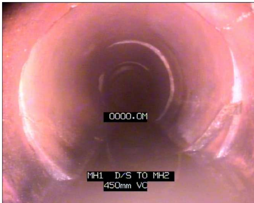
Photo: 1_3A 0m, Fracture, longitudinal, at 2 o'clock
