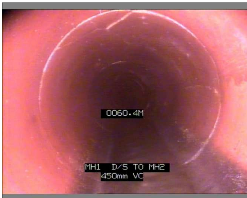
Photo: 1_22A 60.4m, Fracture, circumferential at joint, from 10 to 12 o'clock
