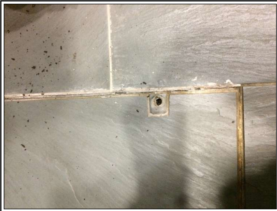
Photo 19, View of MH12 – UTR
