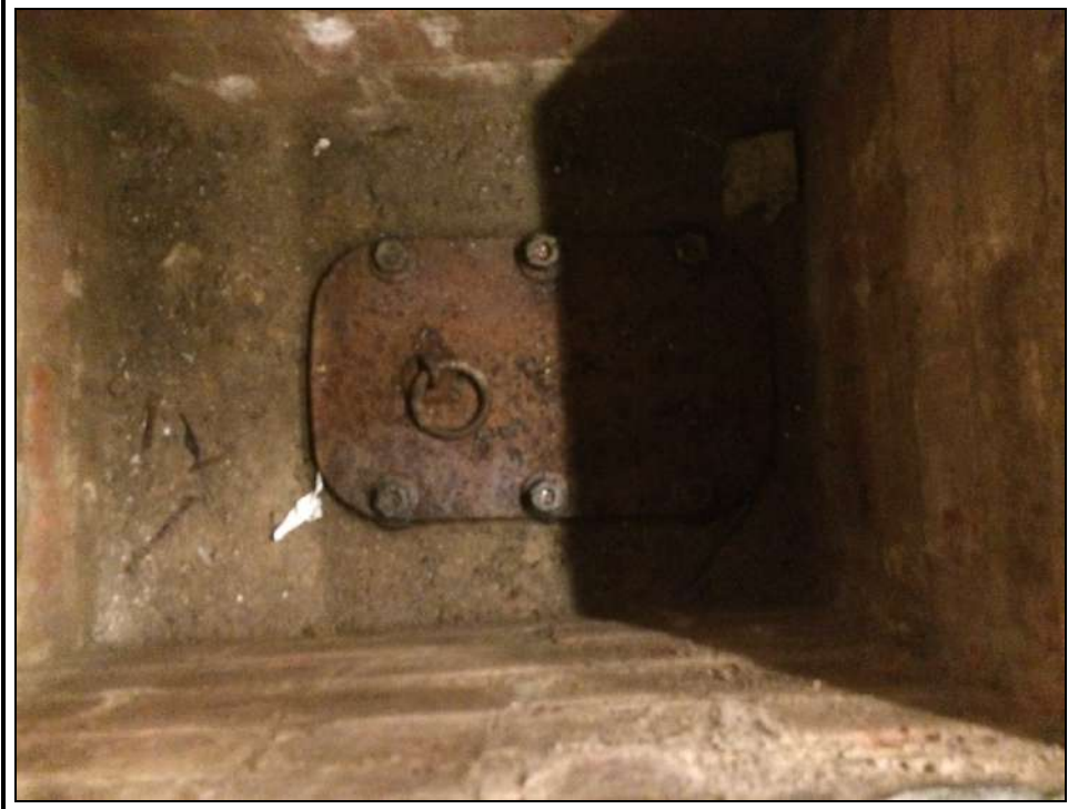
Photo 26, View of MH15 – UTR
