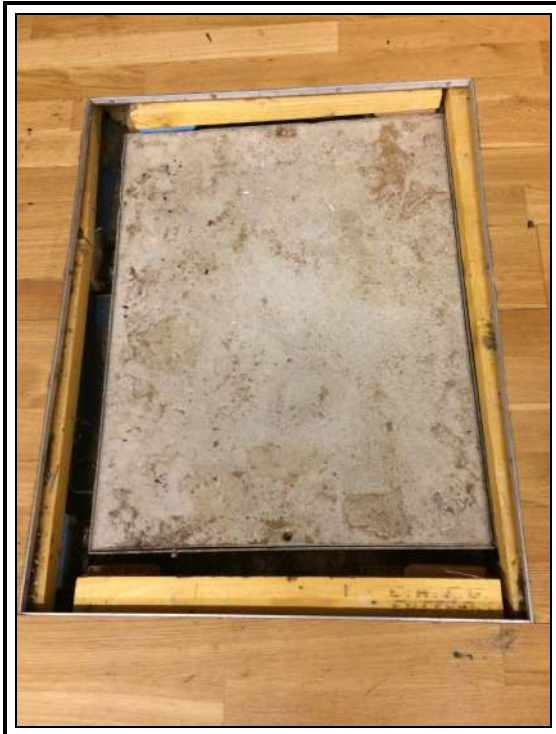
Photo 25, View of MH15 – UTR
