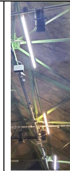
Image 32 Classroom Building, Gymnasium and Swimming Pool - Lighting
