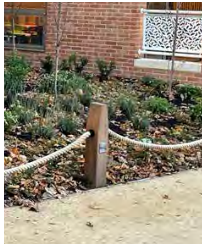
LIGHT BOLLARD AND WALL LIGHT
