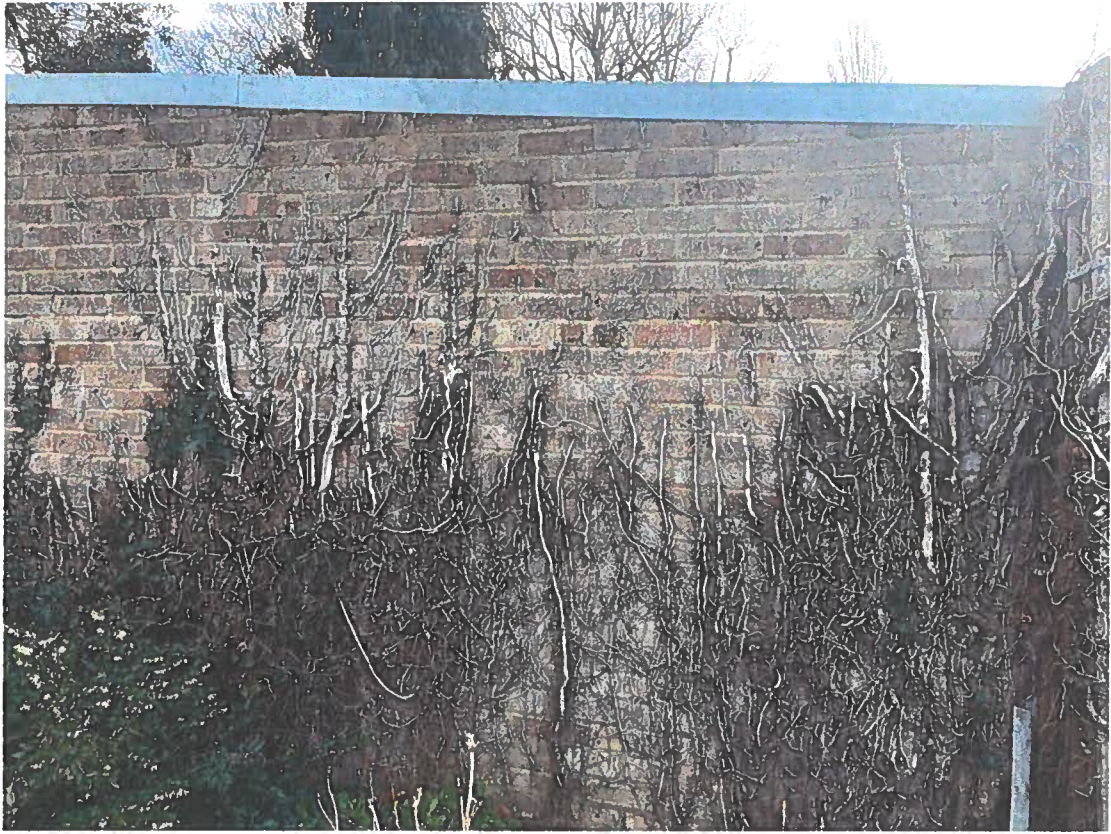
'After' - After image which shows the damaged ivy now
