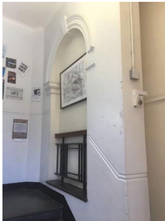
Figure 86. Uncomfortable transition between Science Building and Central Hall. Two adjoining partitions of differing lengths, muddy the plan form within the interior.
