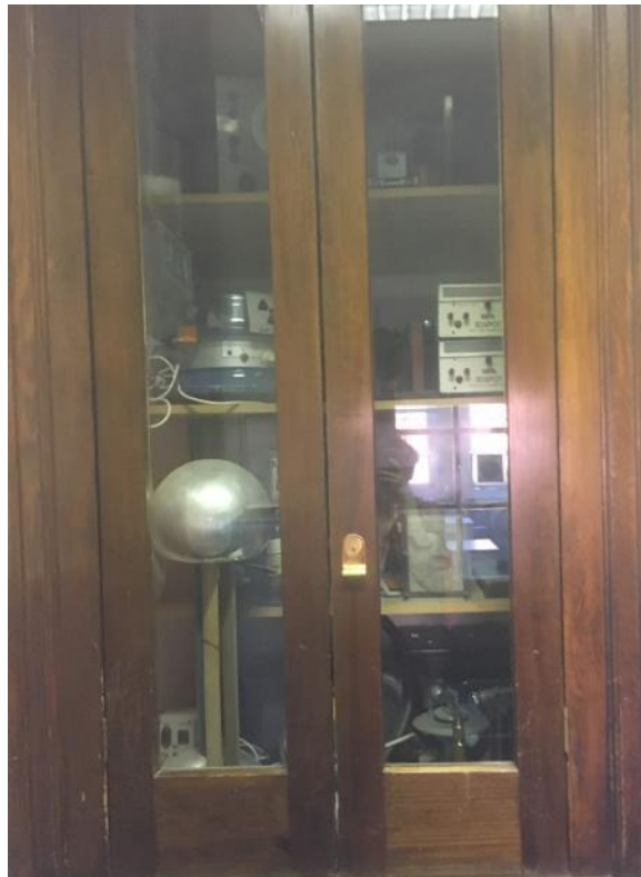
Figure 100. Blocked dumbwaiter within corridor at first floor.
