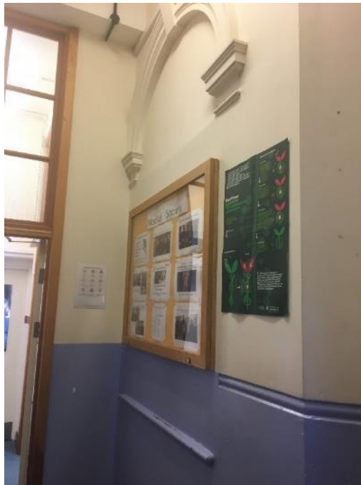
Figure 87. Note unsymmetrical placement of arched moulding, suggesting later alteration.
