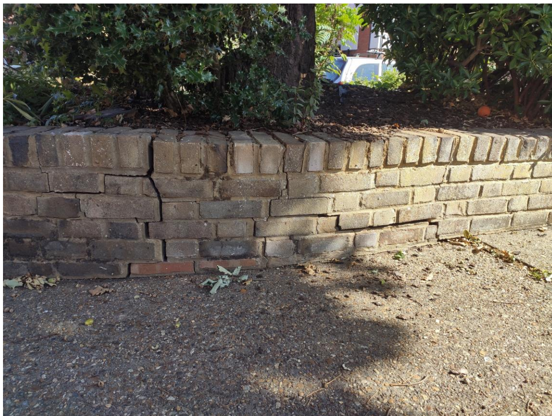
Photograph 3 showing damage to retaining wall of shrubbed at 1 St. Martin's Terrace.
