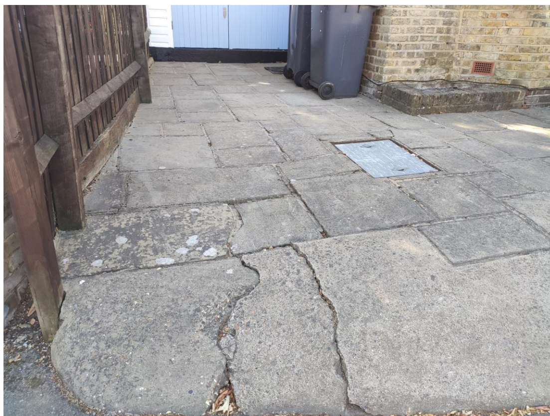
Photograph 6 showing distorted and sunken paving at 14 Page's Lane.
