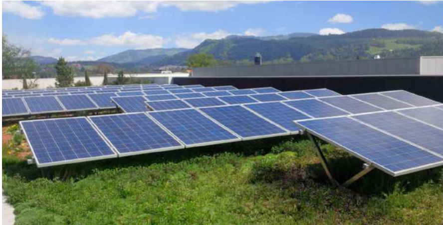
Figure 4: Example of angled PV system on a Green Roof
