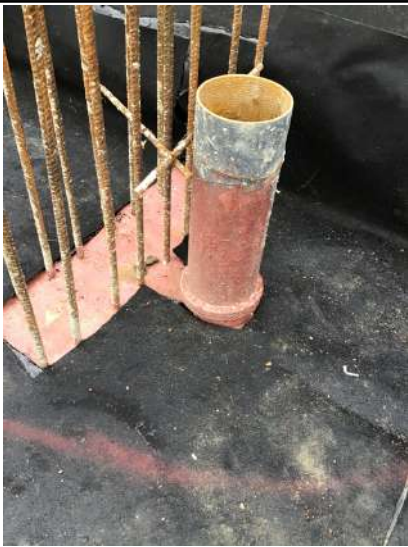
Unsealed pipe penetration.
