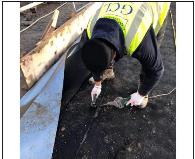
Installers have rectified the gap.
