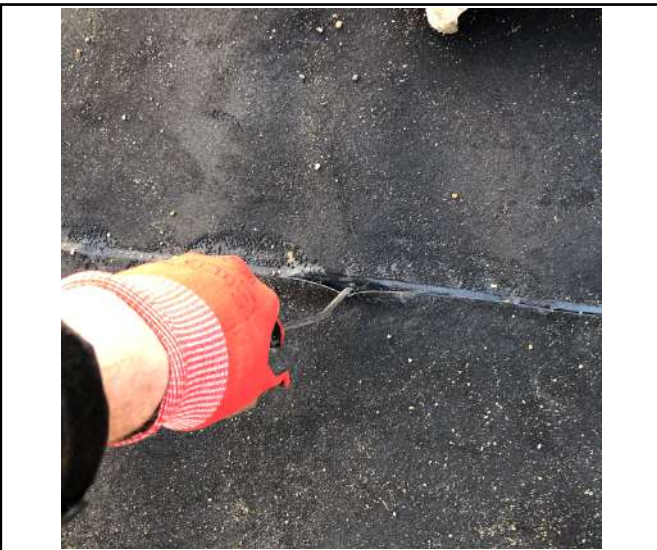
Fault identified in welded lap.
