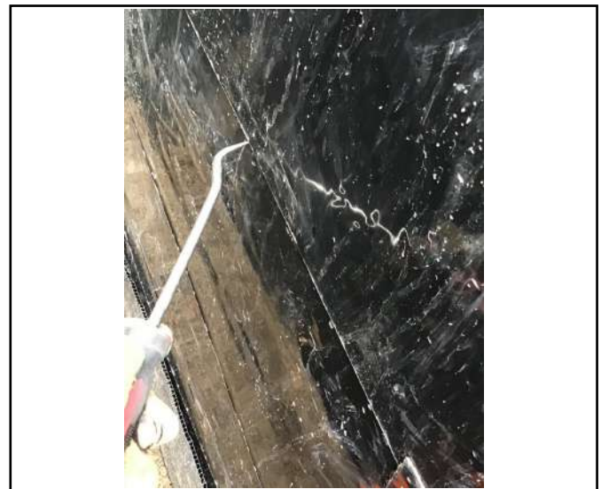
Additional pick and probe test carried
