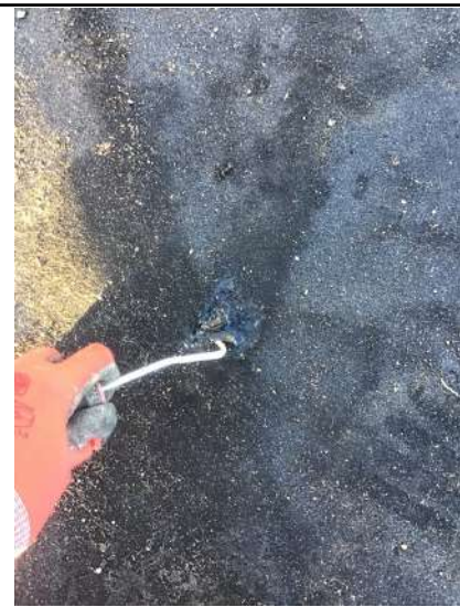
Hole identified in the membrane.
