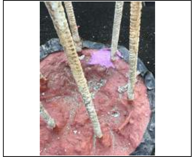
Installers have touched up chip in the
