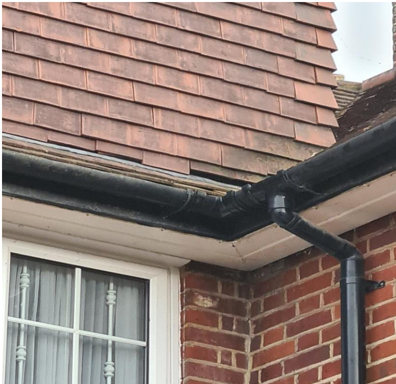
Plate 4: Photograph displaying gaps within the tiles to the front of the property.
