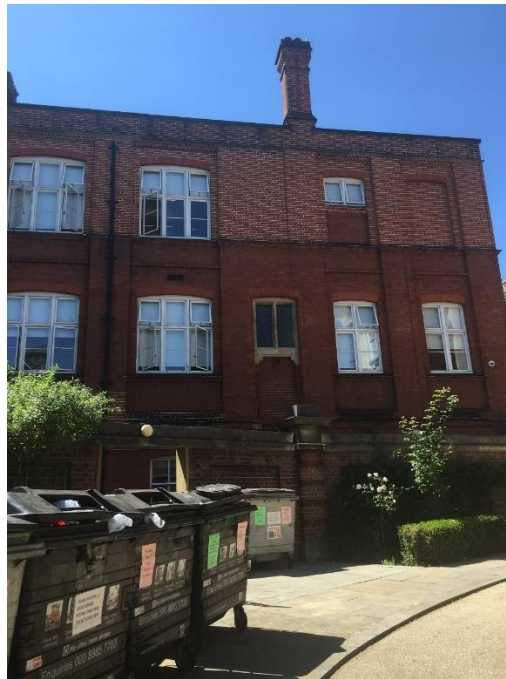
Figure 73. Eastern façade of the Central Hall facing Southwood Lane. Note bins blocking views of the façade as well a single storey brick building which houses a services and WC area.
