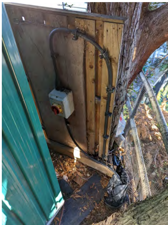
Image 10: Metal-panel shed and associated electric cables in the central part of the site.
