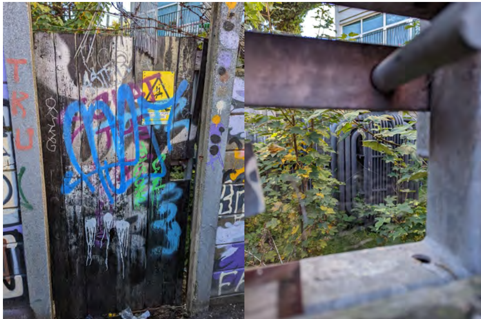
Image 7: Electricity Substation entrance with warning sign obscure by graffiti and the view from the back.
