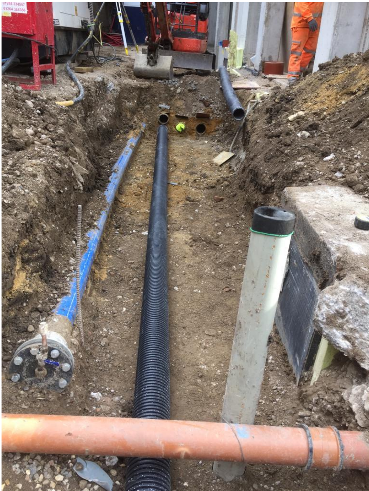
Photograph A4.1 Main water connection showing use of barrier pipe (brown line on pipe).
