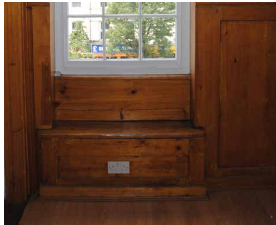
FIGURE 38. Existing Panelling and Skirting
