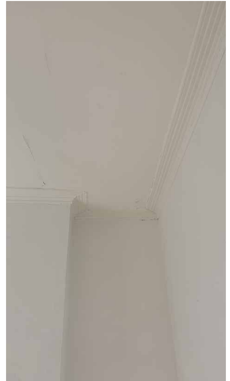
FIGURE 19. Existing Ceiling Cornice
