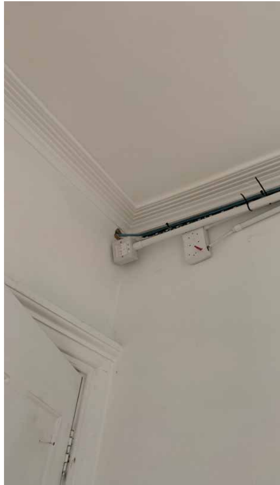
FIGURE 18. Existing Ceiling Cornice
