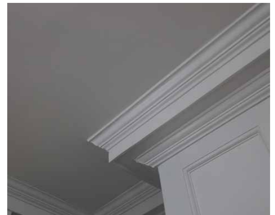
FIGURE 8. Existing Ceiling Cornice
