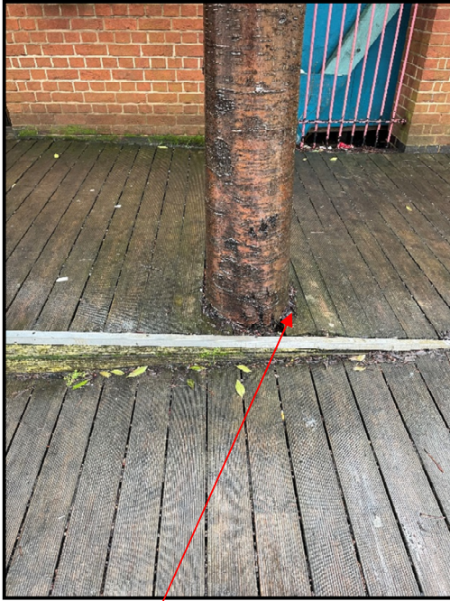
Photo 1: T1 with distorted decking at base
