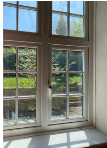
4. Existing plastic windows
