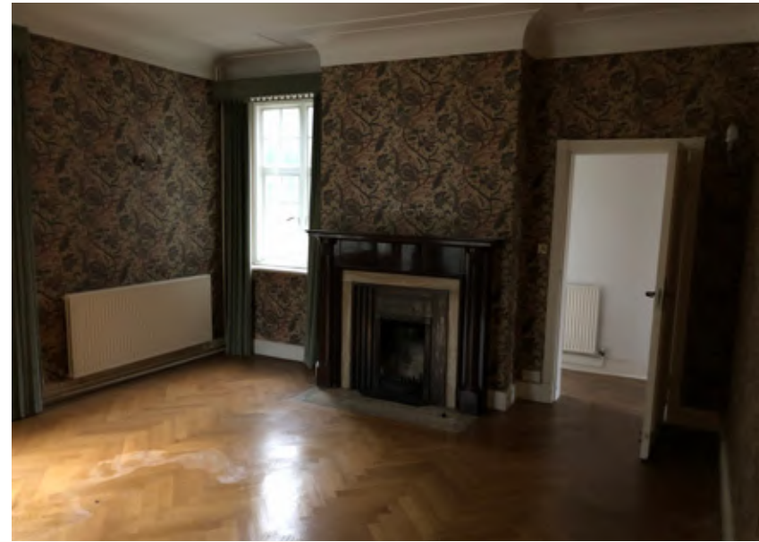
2. Existing dining room - leaking water stains to the floor
