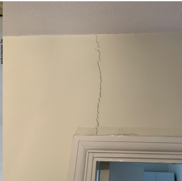
Landing - vertical crack above bedroom door
