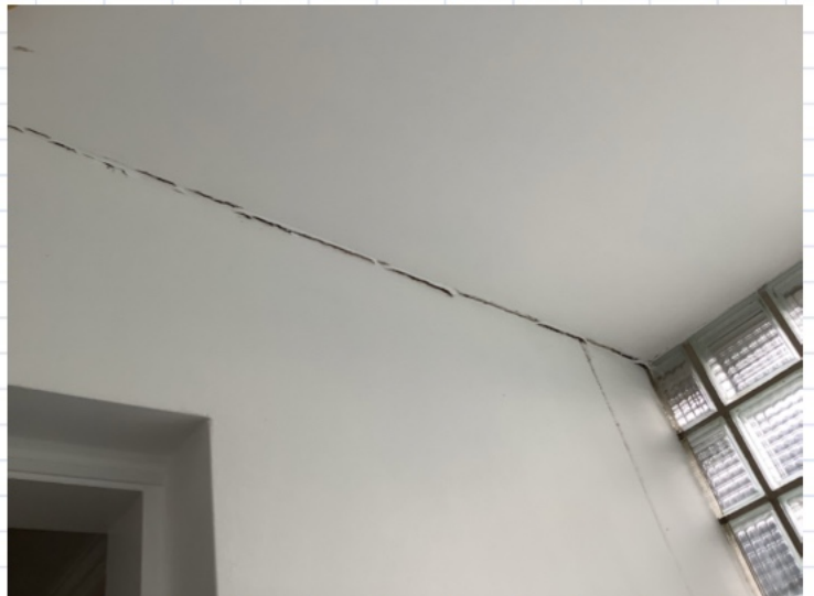
Gap to junction of landing
