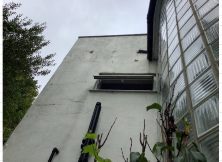
Rear elevation historic render cracks
