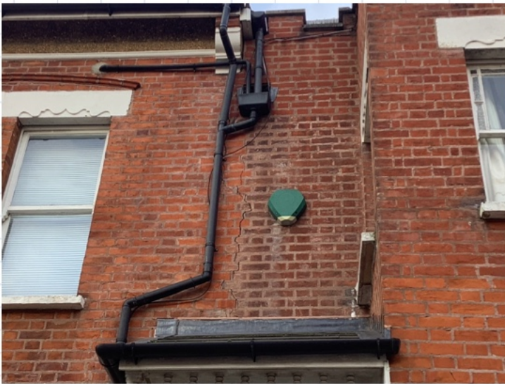
Front elevation crack to line of extension
