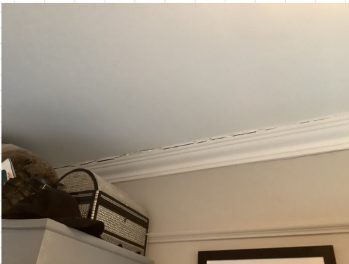
Gap evident to coving in bedroom
