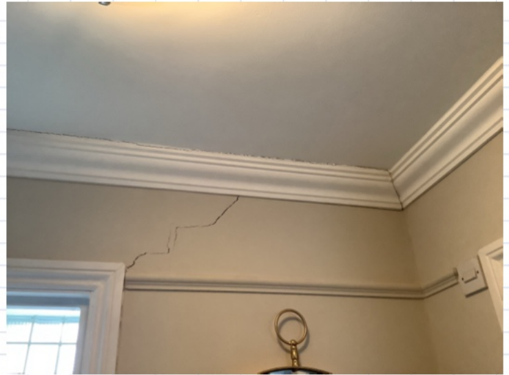
Bedroom wall crack
