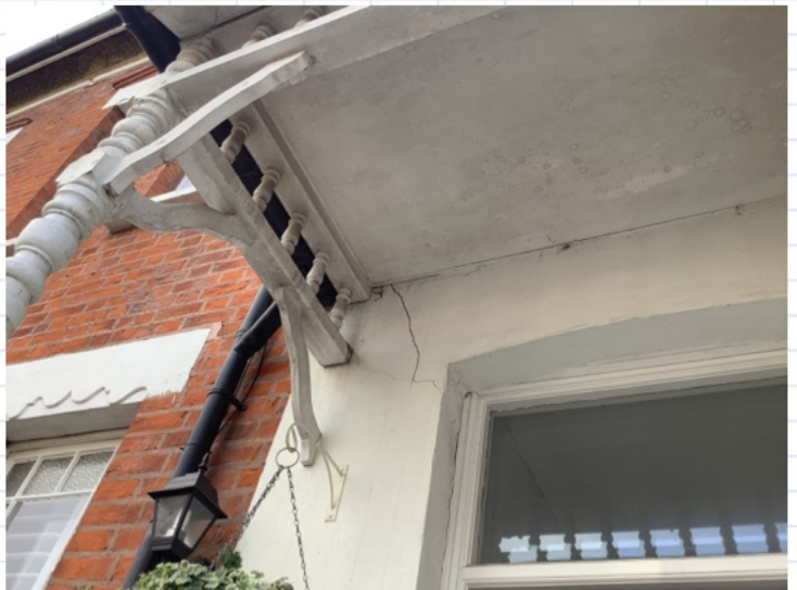
Crack to render above front door
