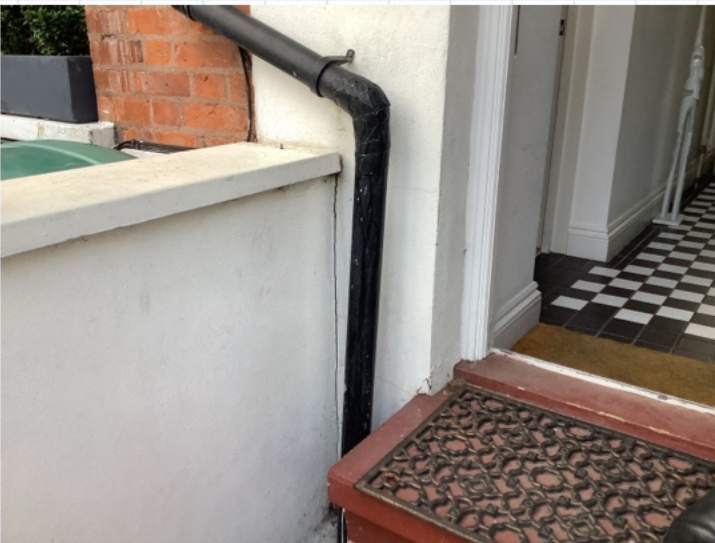
Low level render crack by front door
