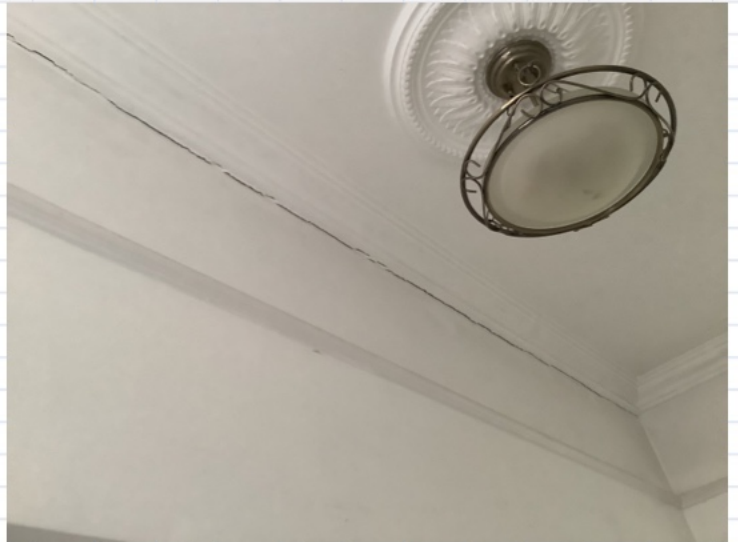
Junction crack to entrance hallway
