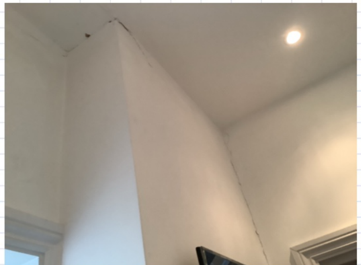
Crack to corridor
