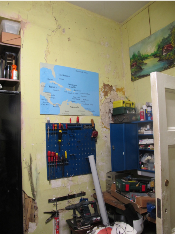
G13 - Moisture damaged plaster to East wall
