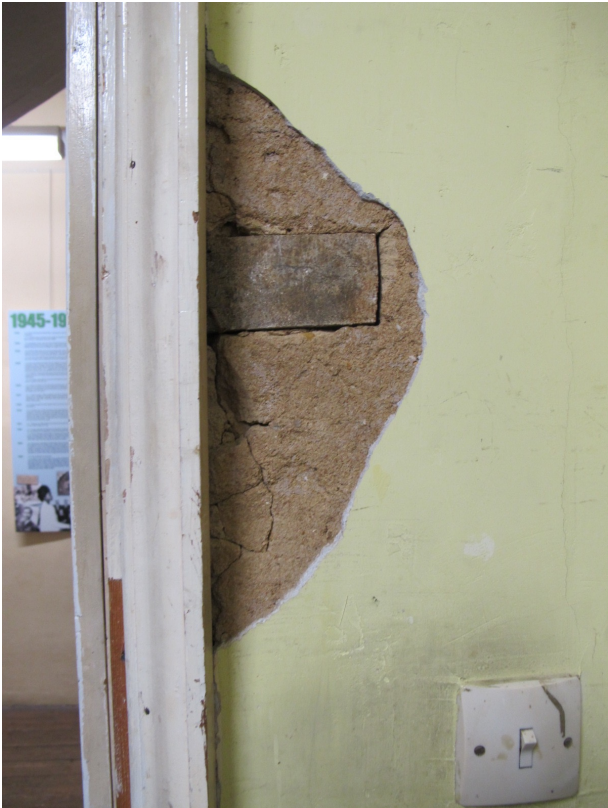
G13 - Missing plaster finish alongside door
