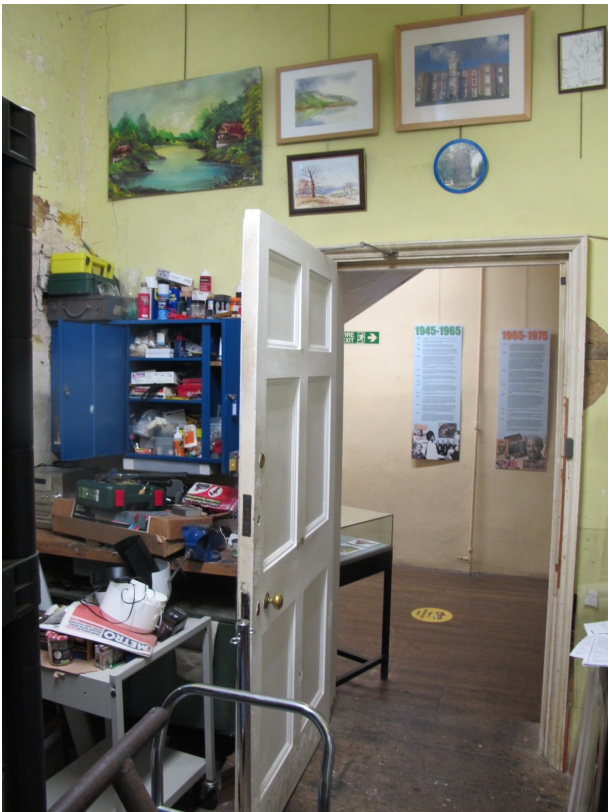
G13 - Moisture damaged plaster to South wall
