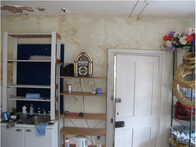
S2 - Water damage to North wall and ceiling
