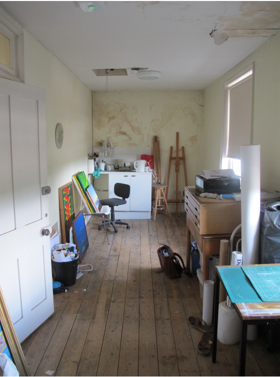
S3 - Water damage to plaster South wall
