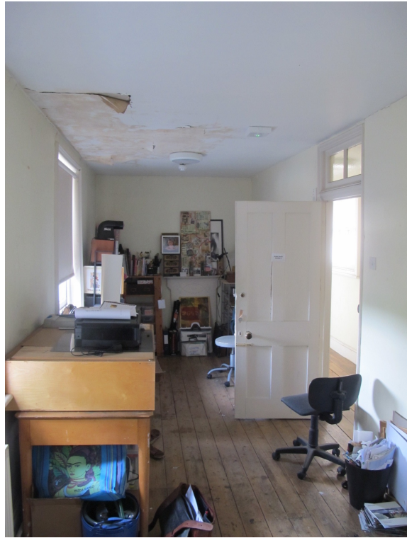
S3 - Water damage to plaster North wall
