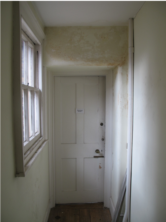
S1 - Water damage to South wall above door to S2
