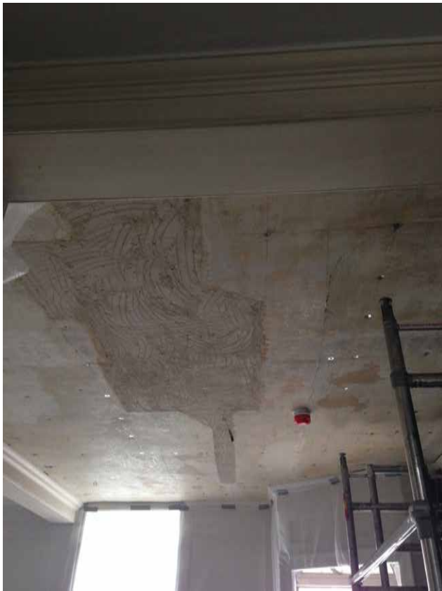
Photo 1 Ceiling area generally with a patch repair
