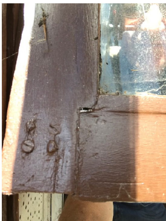
Defective frame corner where there is danger of window failure and consequent danger to persons below from falling glass
