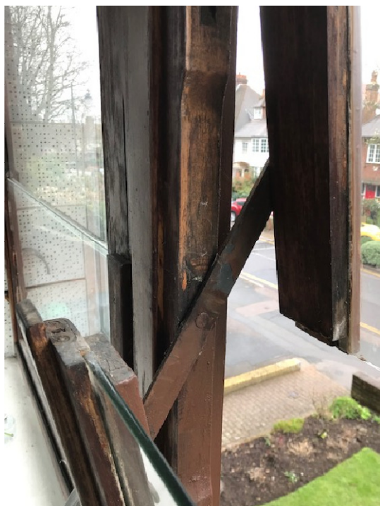
Defective louvre opening operation
