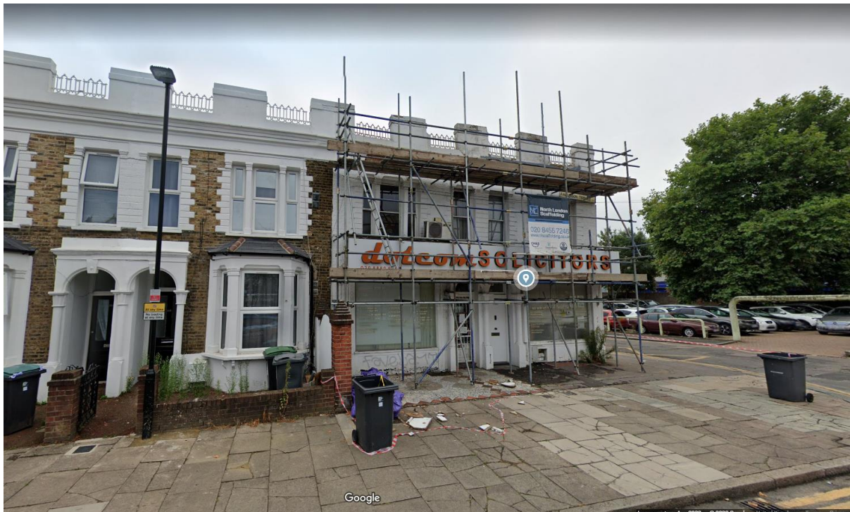
Fig. 2 : Existing front elevation of no. 352 – 354 shows the poor maintenance to the existing façade. A small part of no. 352 is vandalised due to it being left vacant. As can be seen, no. 356 has new UPVc windows installed.
