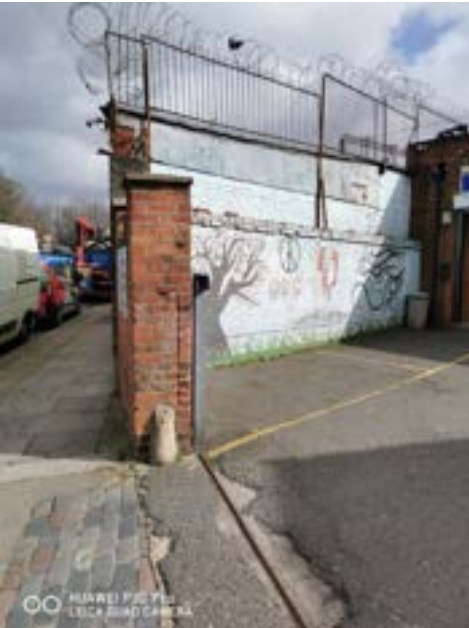
View from the property immediately behind the current dilapidated building to show height of wall and fence above with barbed wire protection.
