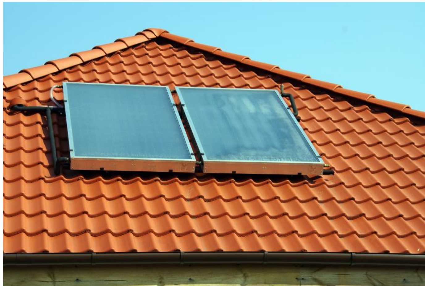
FIGURE 15 –SOLAR WATER HEATING SYSTEM
