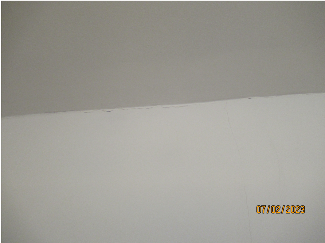
Crack between wall & ceiling in 3
