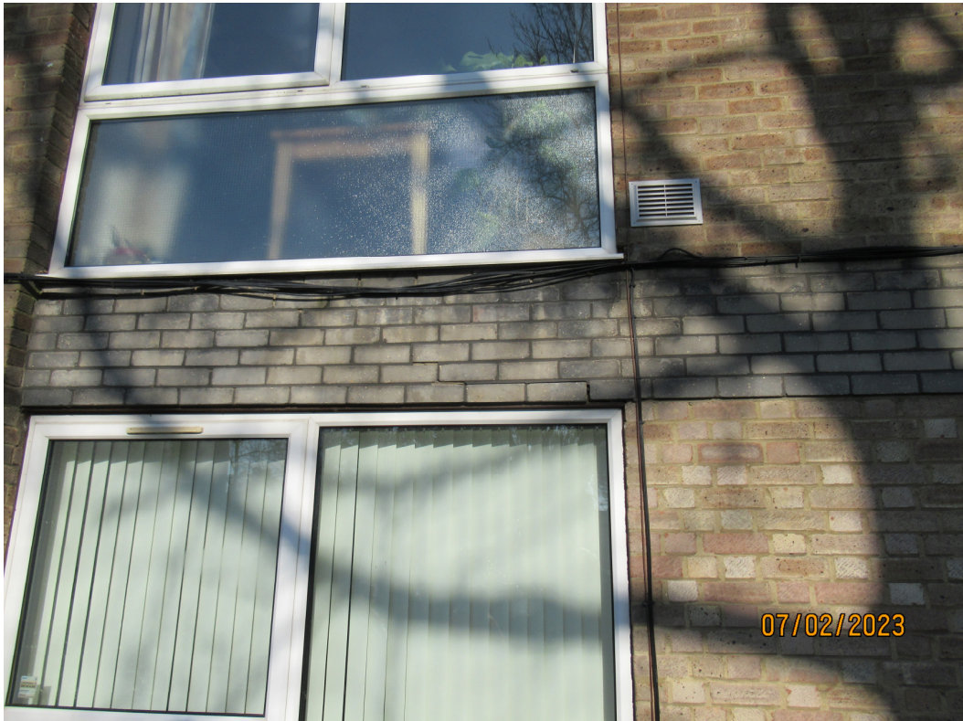
Typical cracking of brick joints above right end of window
