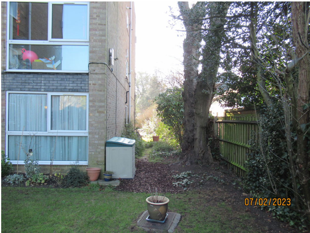
Trees within 3m of west wall, Drain inspection chambers under large terra cotta pots
