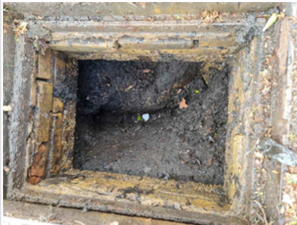
MH/SW - NEXT TO MH7/FL WHICH IS HEAVY SILTED. POSSIBLE COLLAPSE DOWNSTREAM
