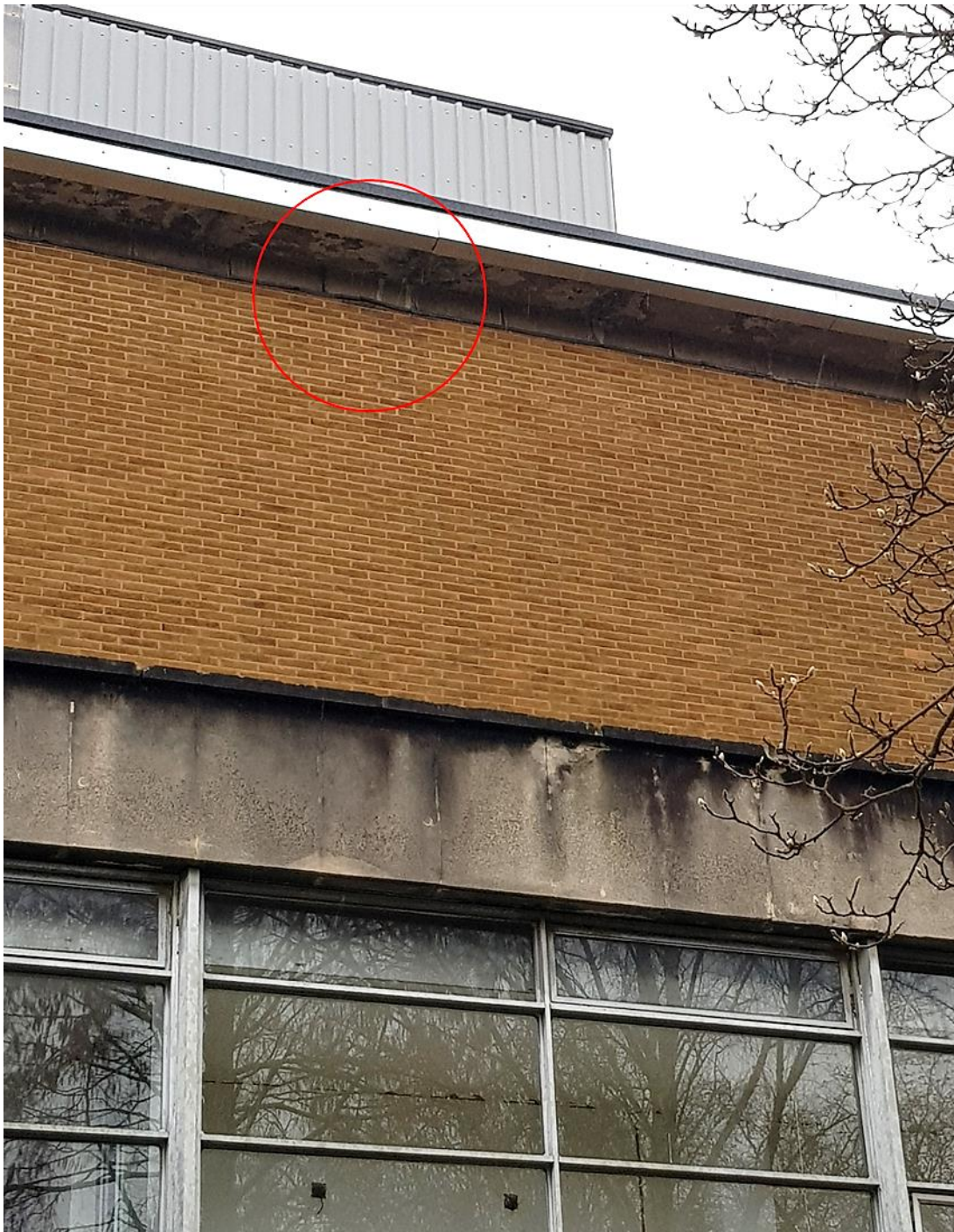
Figure B.13 Features of interest on the buildings: lifted lead flashing, building 1
