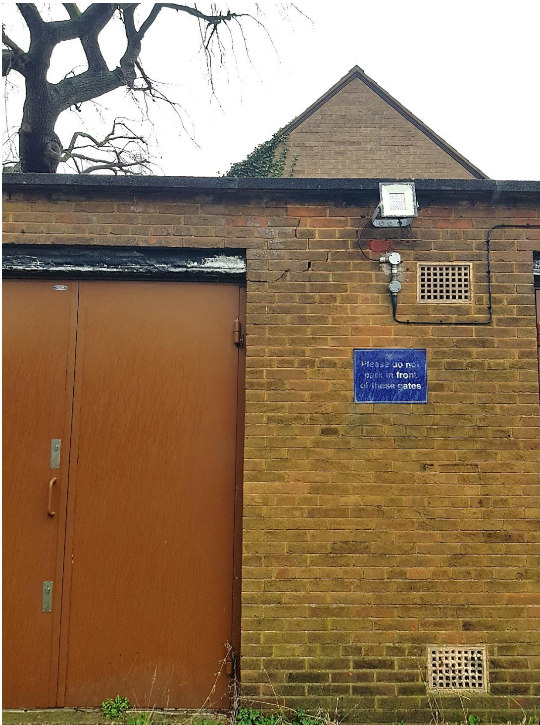
Figure B.14 Features of interest on the buildings: gaps in brickwork, building 2
