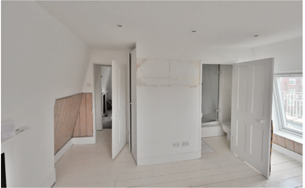
Fig. 42. The modern bathroom enclosure formed within the south attic bedroom with the modern poor quality rooflight providing access to the adjacent flat roof. It is assumed this replaced a historic window.
