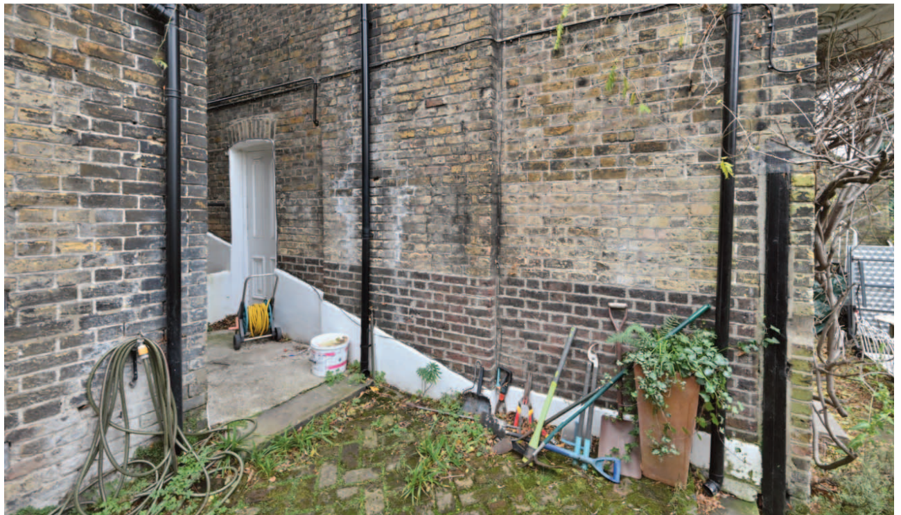
Fig. 13. The former tradesman's entrance with a low wall that extends partly across the steps on the left. This was presumably to prevent water running off the steps into the house. Note the change in brickwork at the base of the wall, and the later cement plinth presumably added as part of damp proofing works.
