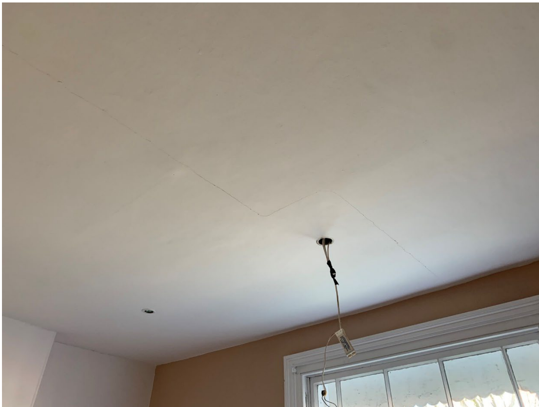
Fig.03 – Evidence of movement in the modern plasterboard ceiling on the street side bedroom
