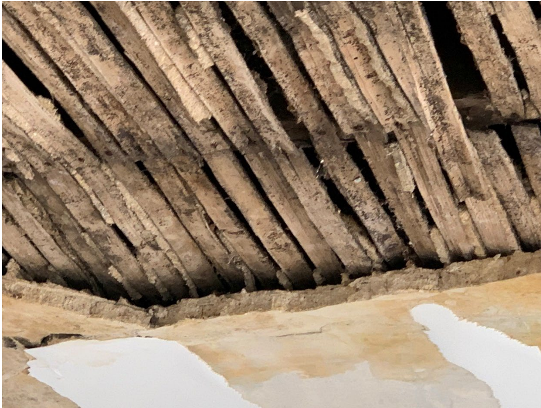
Fig.02 – Sawn oak laths, evidence of corrosion to fixings and broken key between plaster and laths.
