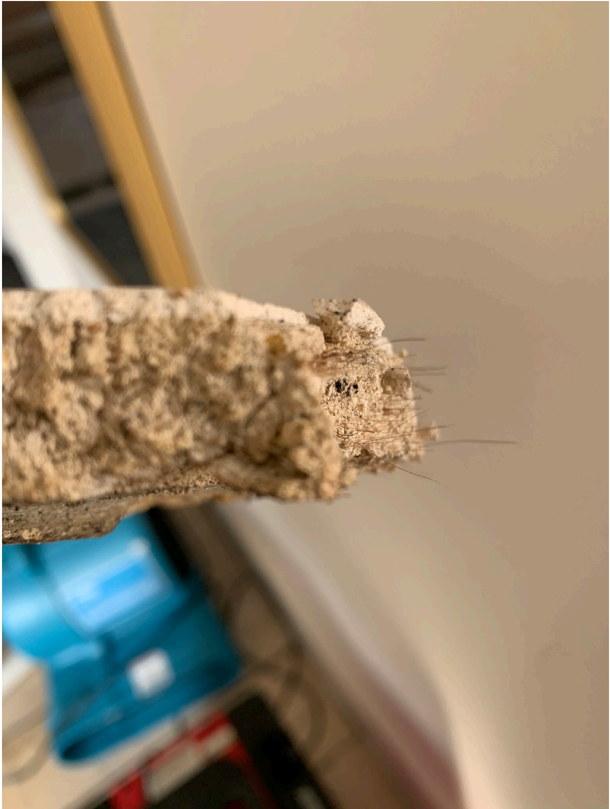
Fig.04 – Detail of existing plaster showing the hair content
