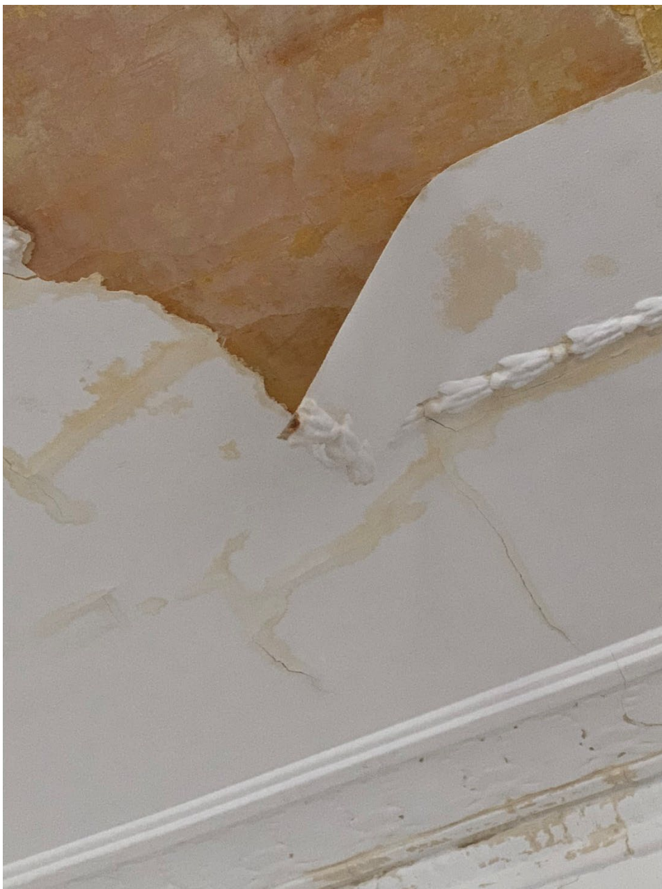
Fig.07 – Water damage to G Floor ceiling. Note the running foliate decoration is not original and is adhered to the lining paper.
