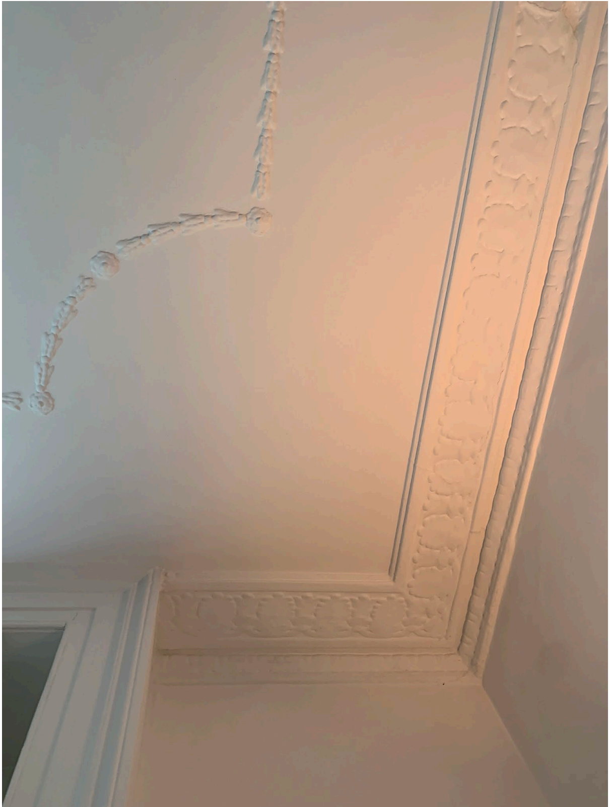
Fig.07 – Pre-flood damage house survey photograph showing original perimeter cornice and modern running foliate detail, both to be replaced to match existing where lost.
