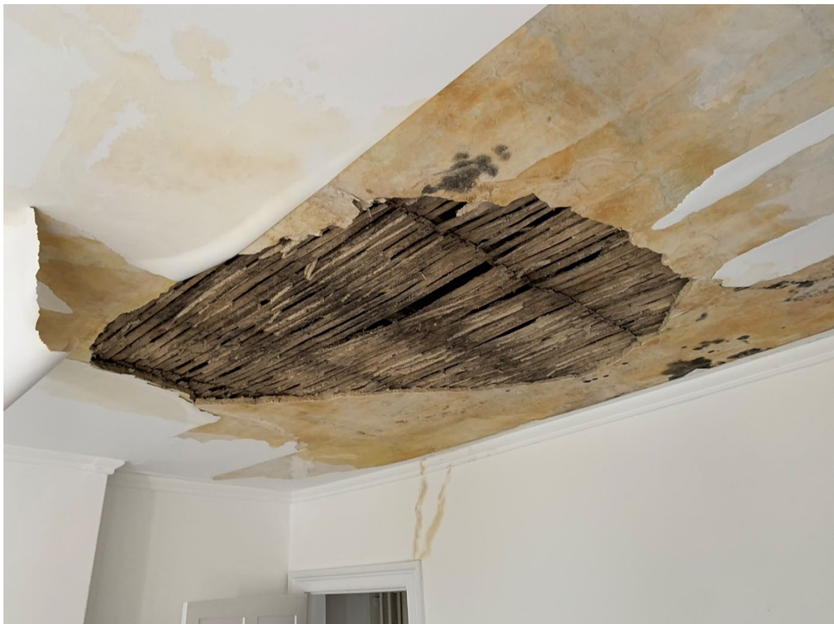
Fig.01 – Area of collapse adjacent to central stairwell.
