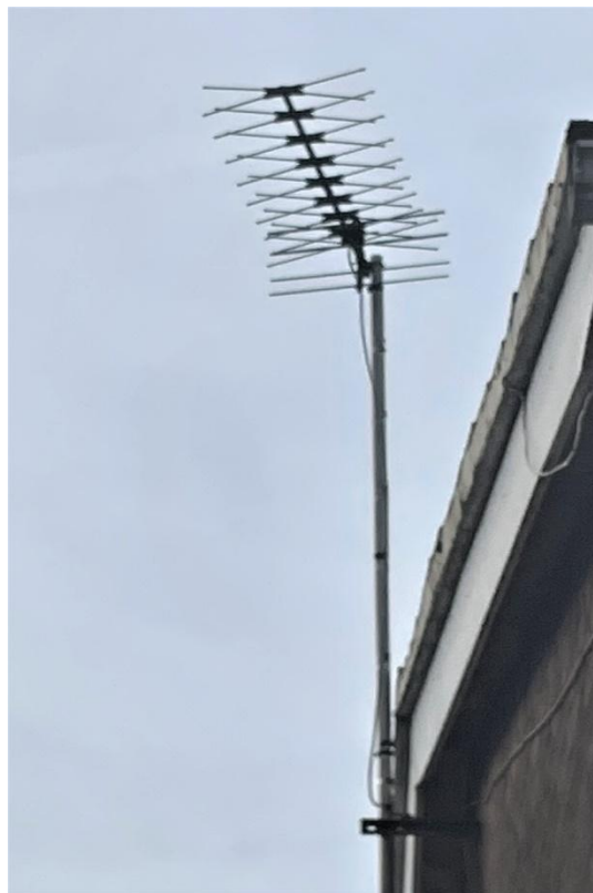
Typical Roof Mounted Aerial Installation
