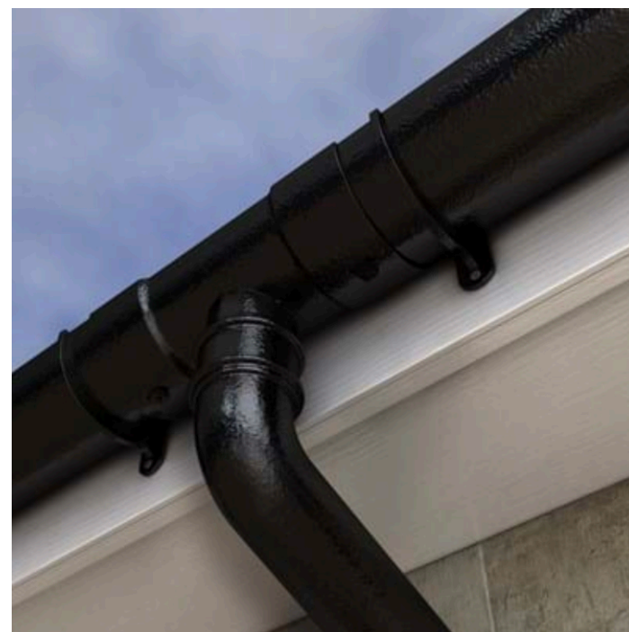
Figures 5+6 (left+top right): Images of original downpipes Figure 7 (bottom right): Proposed cast iron gutter and downpipe
