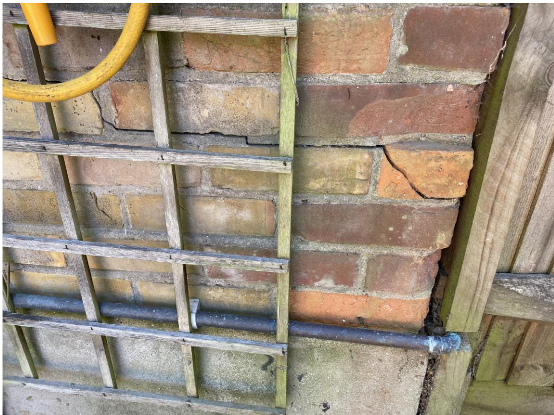
Photo 2 Low level cracks rear left corner
