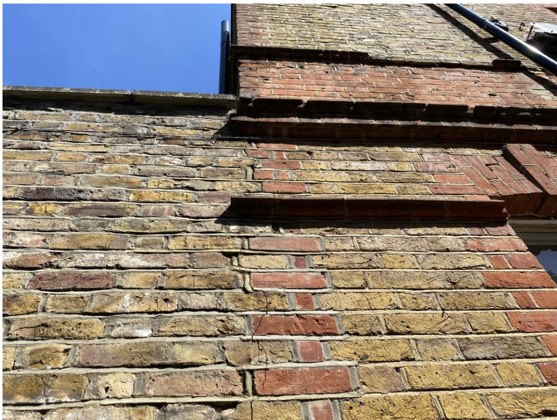
Photo 3 Cracking to left wall at junction with main house
