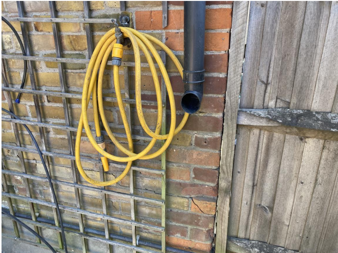
Photo 7 RWDP and outside tap rear left corner
