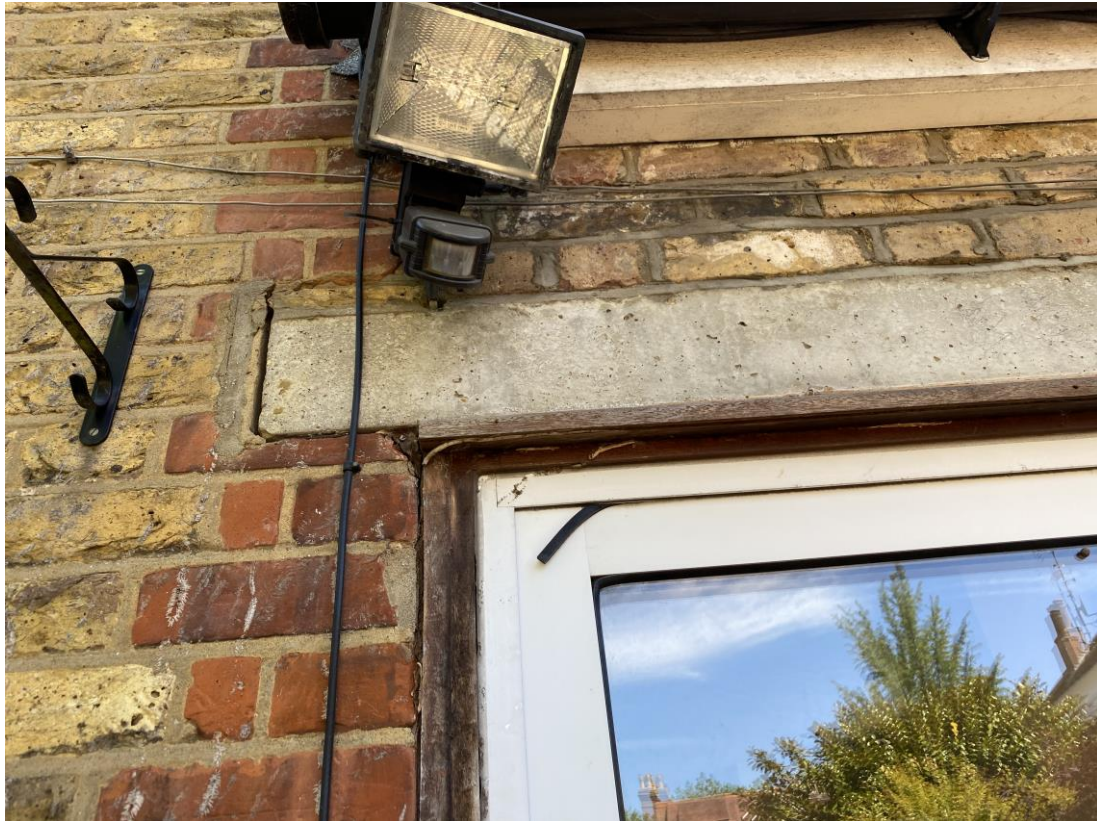
Photo 1 Cracking over rhs kitchen door
