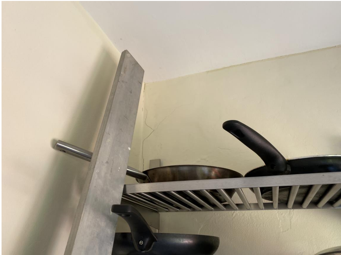
Photo 5 Cracking left wall
