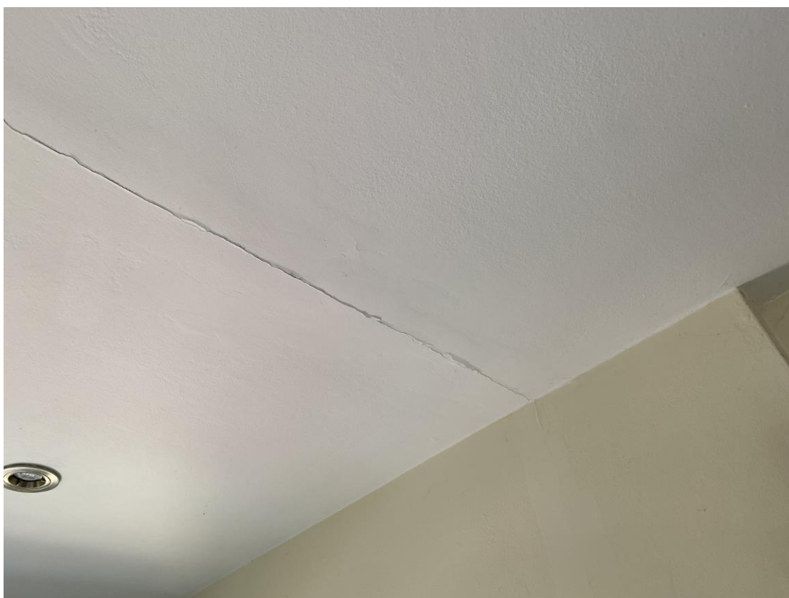
Photo 4 Kitchen crack across ceiling
